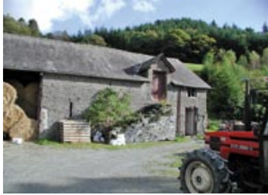
Mass concrete construction on the Plas Dinas estate Adeilad mâs-concritid ar ystad Plas Dinas
